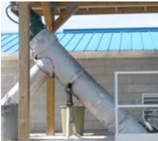
Cold Weather System Insulation Blanket
