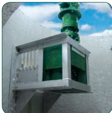
Mini Monster installed in a pump station
