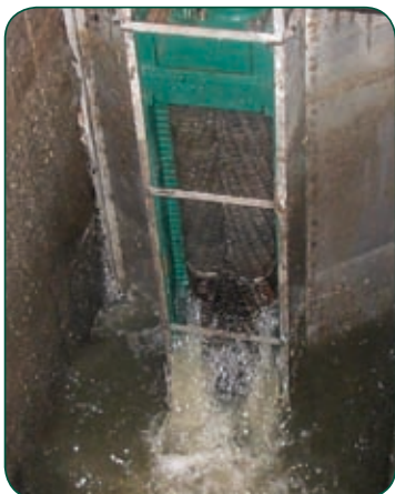
Muffin Monster in pump station
