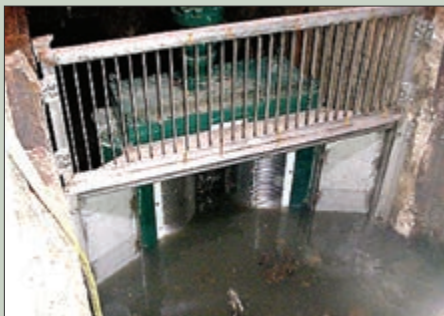
Overflow bar screens
