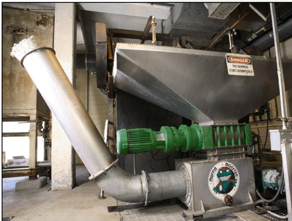
Captured solids are ground into small particles then cleaned, washed and dewatered before being pushed out the exit chute as clean, dry disposable waste.
