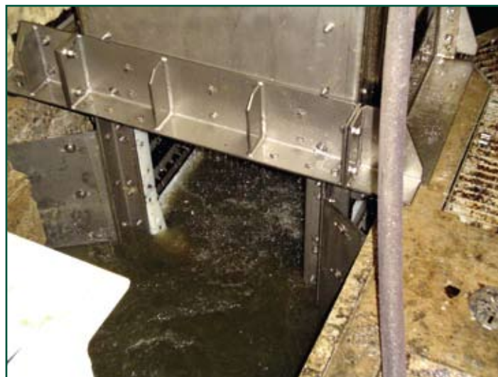
The Monster Separation System keeps the facility’s treatment processes safe and trouble free.
