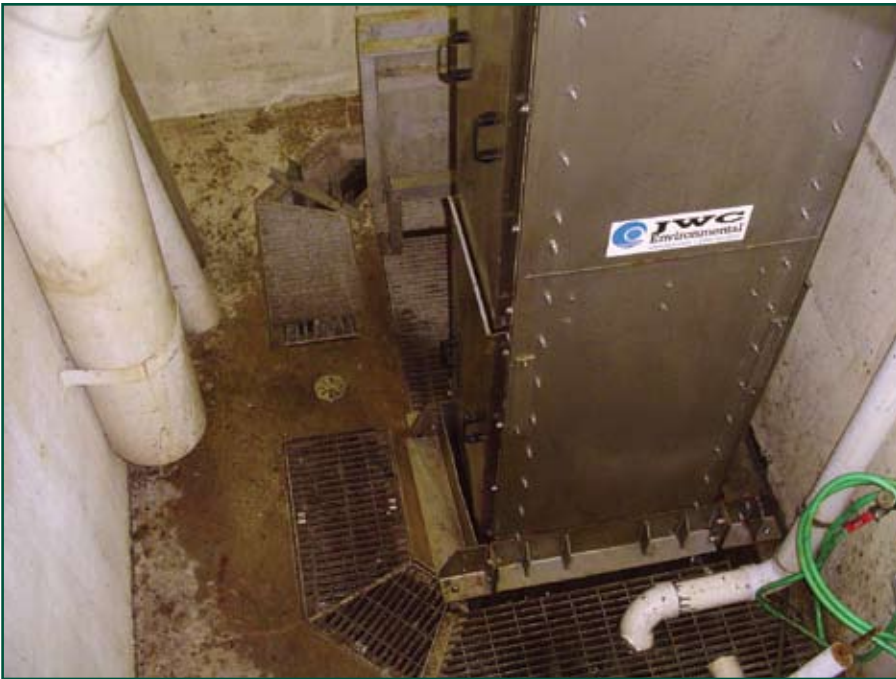
The Bandscreen Monster's inside-out flow pattern keeps the surrounding areas clean while lifting captured solids to the Screenings Washer Monster.
