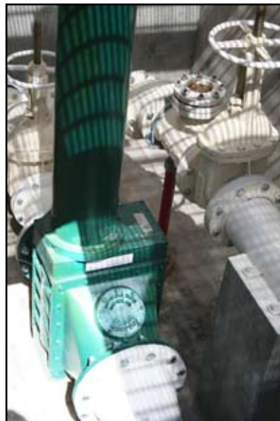
This Macho Monster is located in an underground vault where sewage from the jail passes through it and into the city sewer system for treatment
