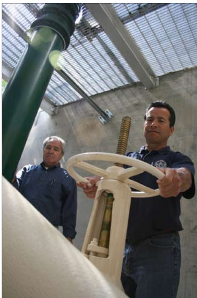
Jail facility managers Harry Mira (left) and Robert Rocho (right) stand next to the Macho Monster.
