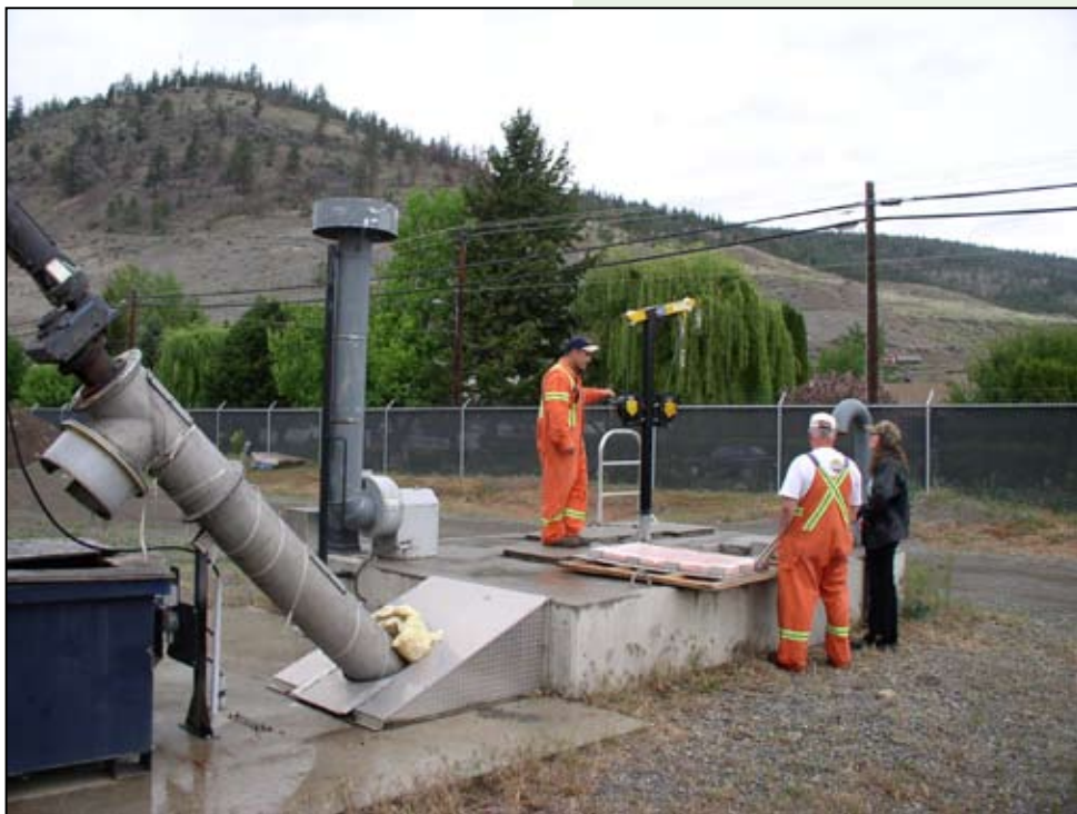
Processed screenings are conveyed up the Auger to a trash receptacle.
